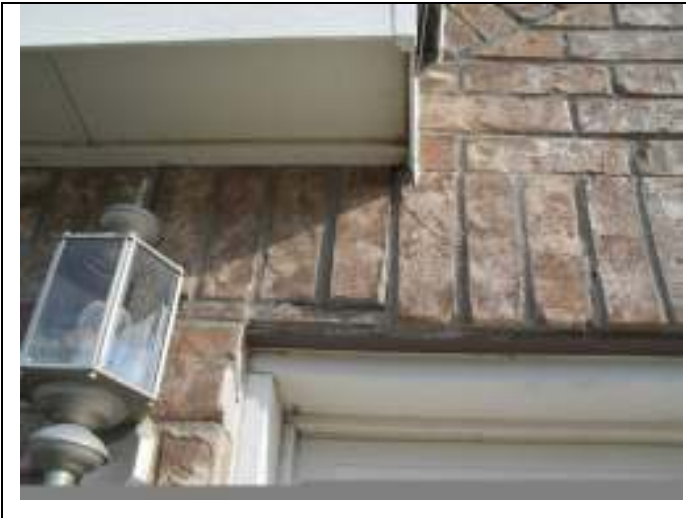
Sample of exterior brickwork crack
