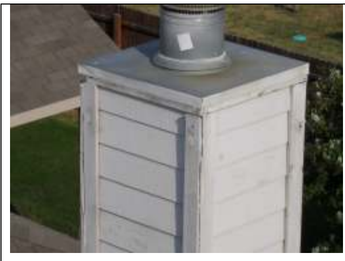
Sample of damaged and separated trim at chimney
