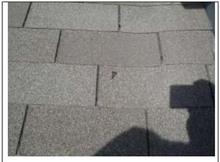
Sample of exposed nail in the roof
