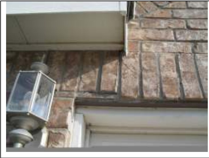
Sample of exterior brickwork crack
